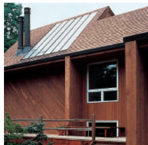
■ Figure 27-5 The solar panels on this building use the photoelectric effect to convert the Sun’s light to electricity.
