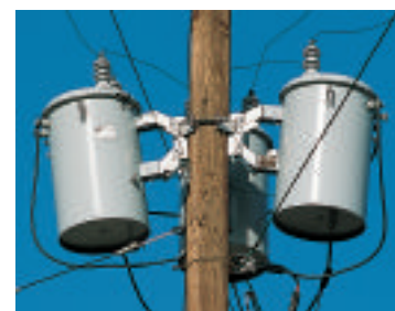
■ Figure 25-15 Step-down transformers are used to reduce the high voltages in transmission lines to levels appropriate for consumers at the points of use.
